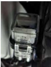
x2 heater fuses under plastic cover
