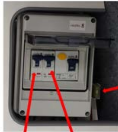
Sargent Charger 240v Sockets in kitchen
