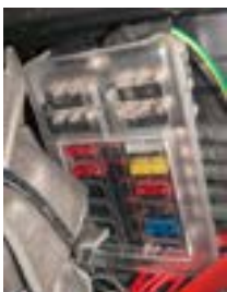
Fuse board - heater fuse is the white 25A
